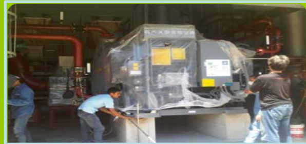
Waste Incineration Plant – Sainoi, Nonthaburee Model: BDE20 Cooling capacity: 39RT Fuel: Exhaust Gas from Waste Incineration
