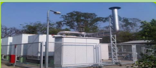
PTT, Chonburee Model: BYZ20 , BCT115, BCTDE70 Fuel: Direct Fired (NG) , Exhaust Gas from Micro Turbine Cooling capacity: 60RT x 3 sets + 33 RT x 2 sets + 20 RT x 1 set
