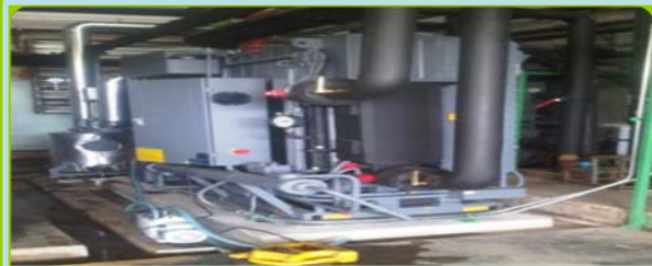
TUC Elastic Co.,Ltd., Prachinburee Waste Heat Recovery from Hot Oil Boiler to Air-conditioning System Model: BDS20 Cooling capacity: 60 RT
